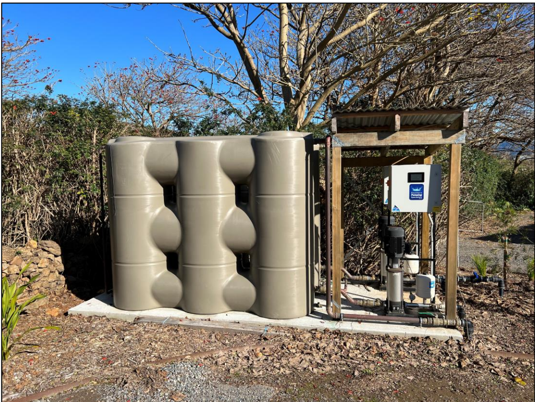
Site Photograph 6.7.2 Aboveground storage tank observed on the southern boundary of the site, adjacent the driveway, viewed facing south.
